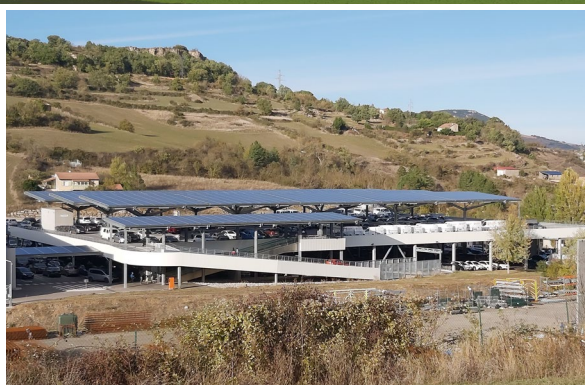
Ombrière de parking, Creissels (12). © Étienne Louyriac
